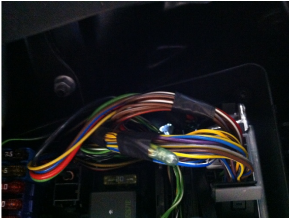
Wire Route (Fuse box side)
