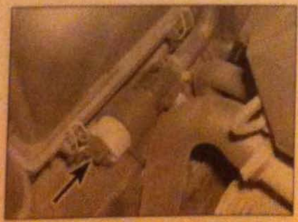
10.30 Main supply valve, seen from above with air cleaner removed - wiring plug arrowed
