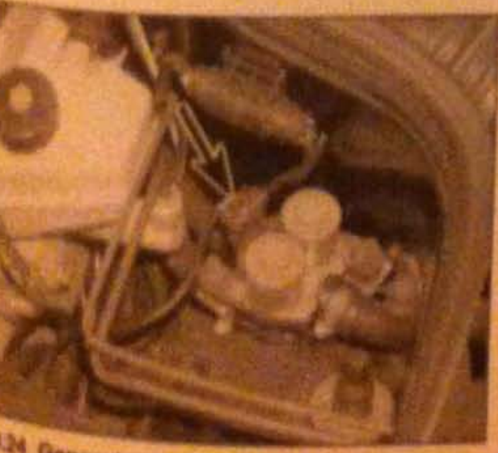
10.24 General view of the solenoid valves - wiring plug arrowed
