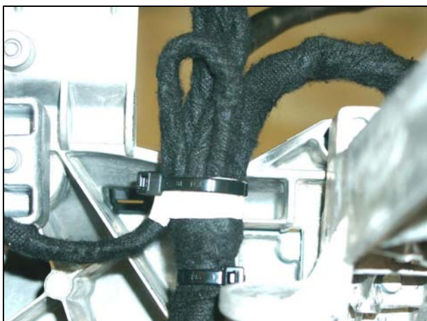
Figure 12 P-B-91.60/99c Repair loop cable tied to cockpit harness (Repair up to MY 04)
