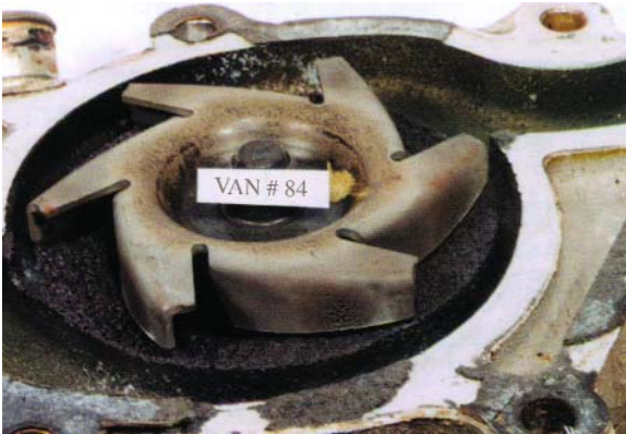
This coolant pump chamber was pockmarked by cavitation erosion-corrosion, which would eventually reduce performance of the pump.
